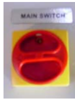
Turn on "Main Switch"
